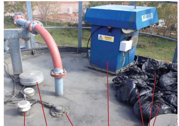
Level probe PRV Pressure sensor Air filter Bags of leaked product
