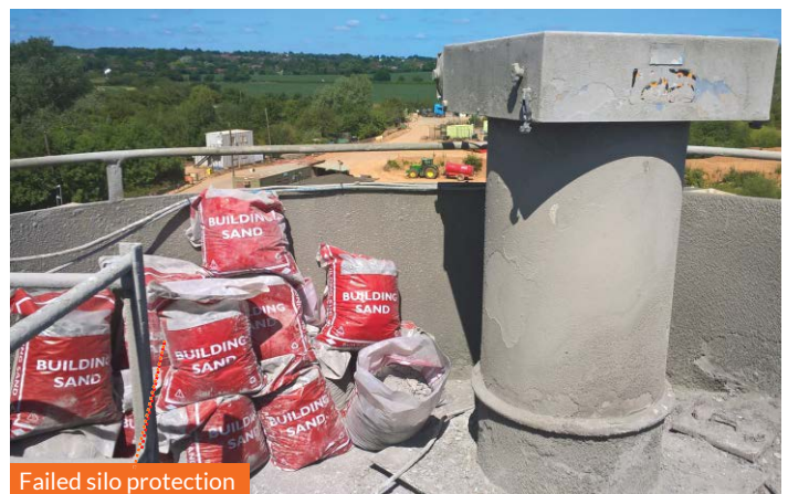
Failed silo protection
